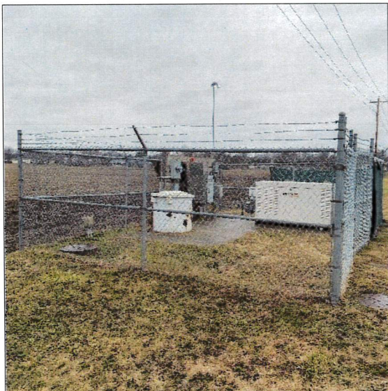
Figure 1 - Highway Lift Station
