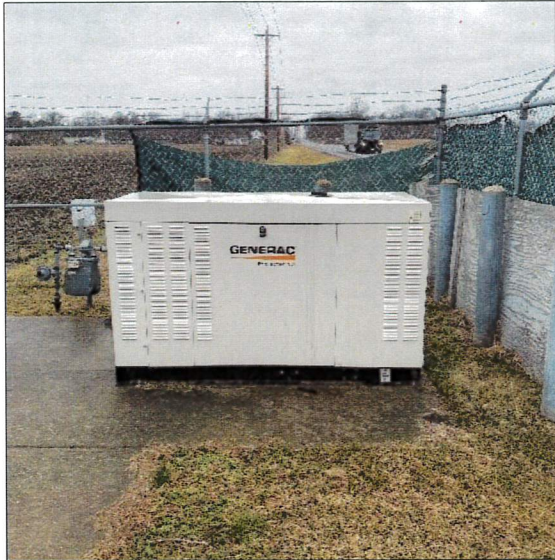
Figure 3 - Highway Lift Station Generator
